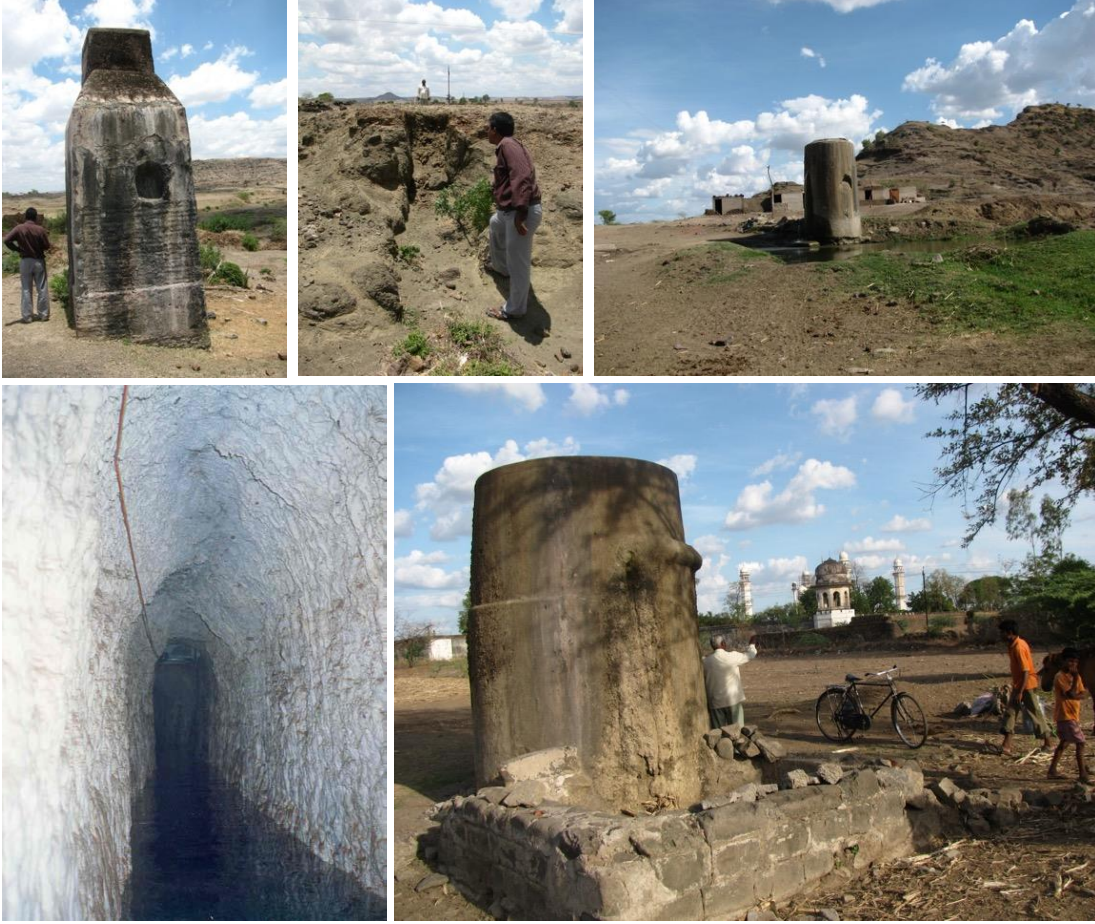
Fig. 35: Manholes of the naher system of Shambhaji Nagar (Aurangabad)
